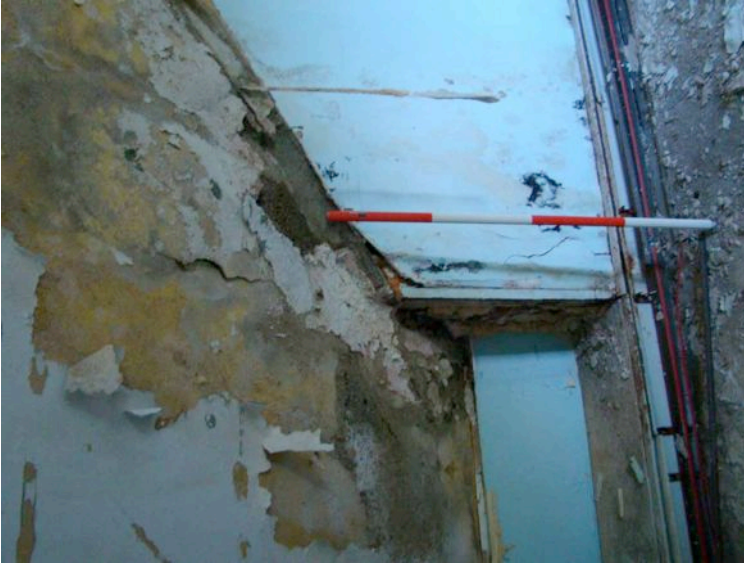
Over Archway: Water damage.
