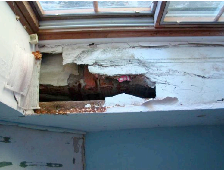
Over Archway: Water damage.
