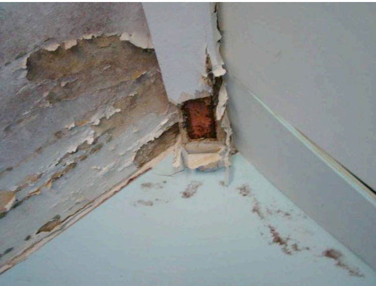
Over Archway: Water damage.
