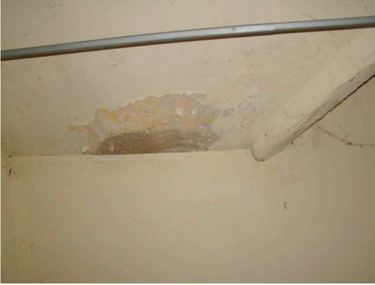
Over Archway: Water damage.
