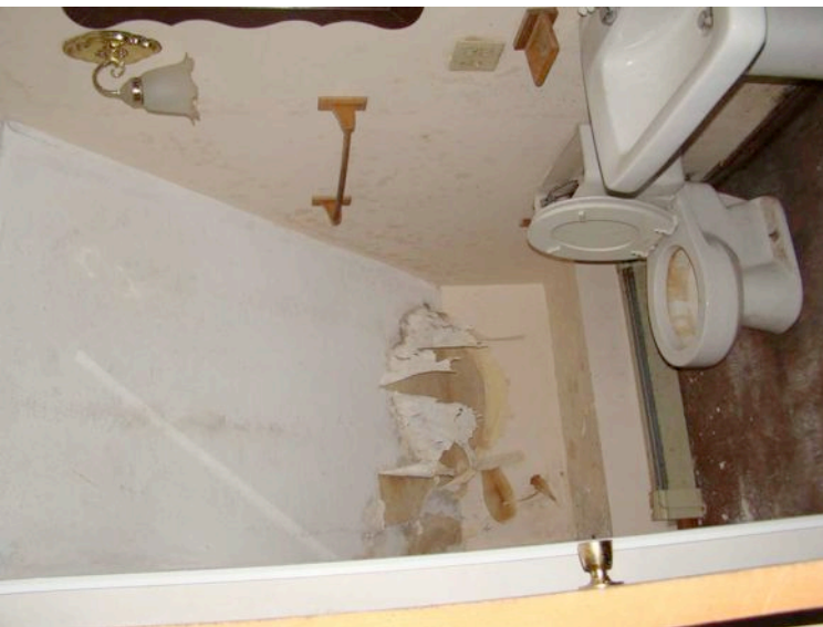
Over Archway: Water damage.
