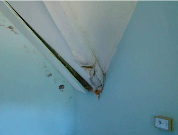
Over Archway: Water damage.
