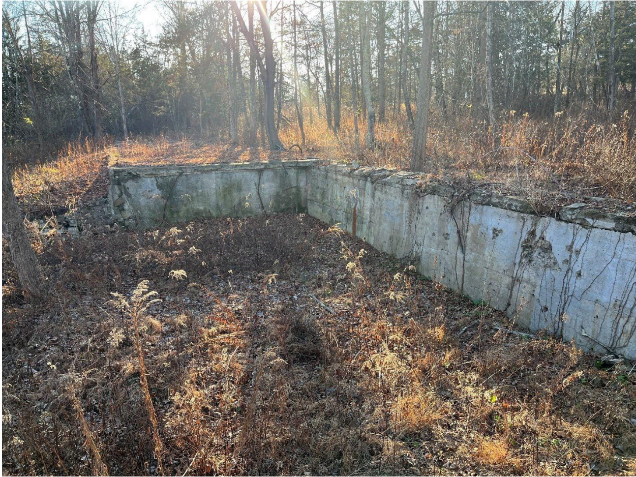
Image 22- Exterior, view of former farm building's concrete foundation outline located on the edge of the property. It is likely this building was used by Kauder when it functioned as a large scale chicken farm.
